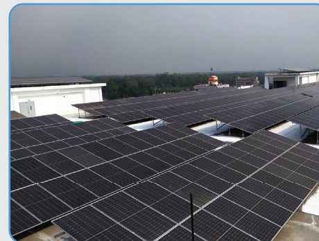
Commercial and Industrial Rooftop Solar Solution
