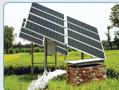
Solar Irrigation Pump
