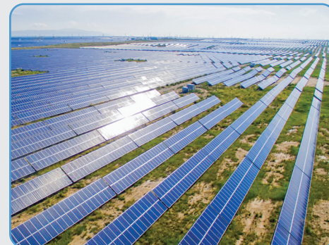
Solar Power Plant
