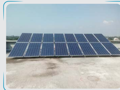
Residential Solar Setup
