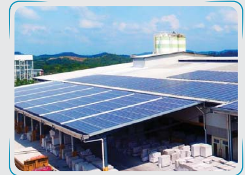
Commercial/Industrial Solar Setup
