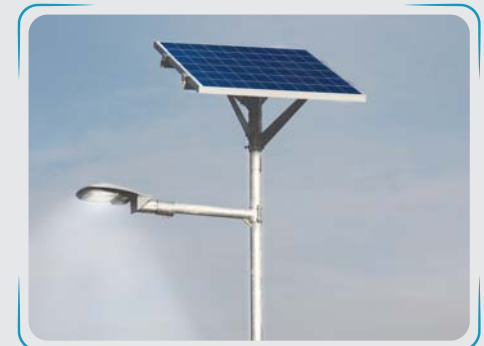
Solar Street Lighting
